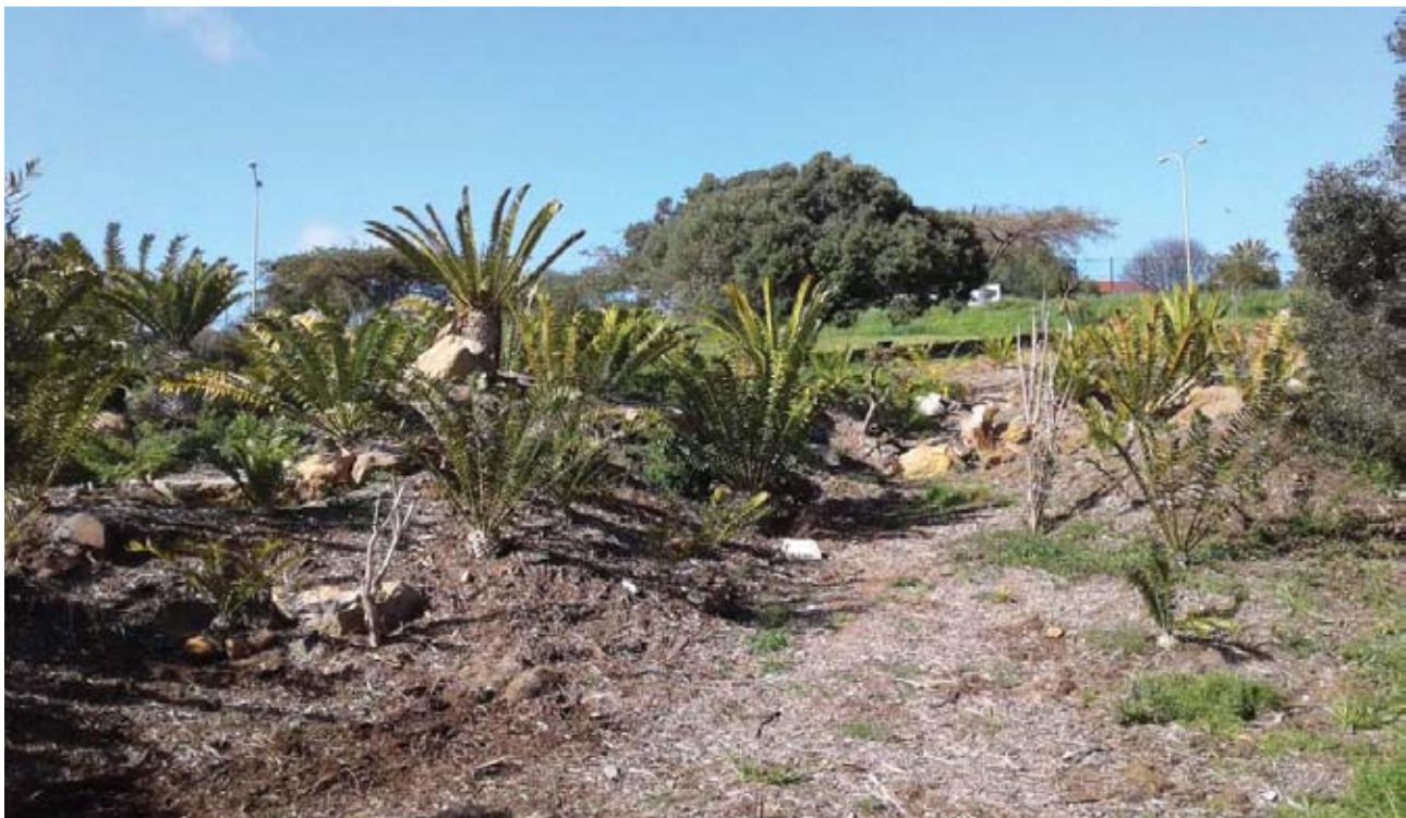
Figure 2. A little "valley" was created by moving soil and adding huge rocks to the sides to stabilise the slopes. This should improve drainage and provide a happy home to the cycads.
